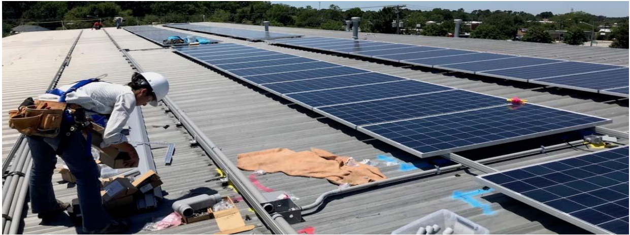
Figure 1: Installation of PV system on the roof of the commercial facility (source: www.carolinasolarquote.com )
